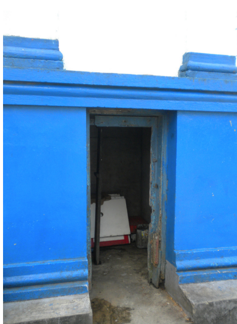
Entrance Door Non Existent
